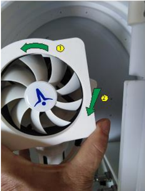
Figure 10: Removing the fan housing with the fan (magnets) and clean it with brush
